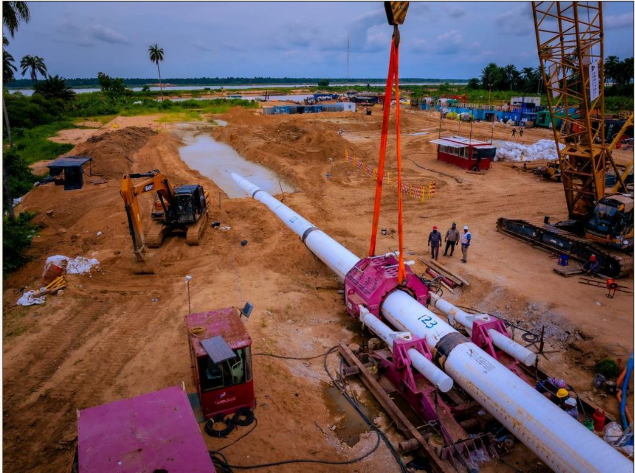
Pipeline Infrastructure — Engineering Across Nigeria's Energy Network.
