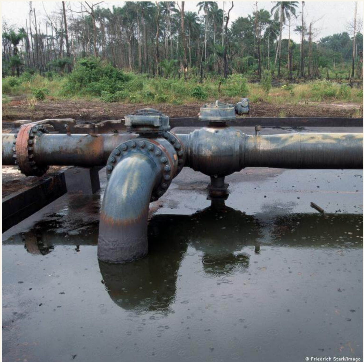
Oil pipeline infrastructure in the Niger Delta.
